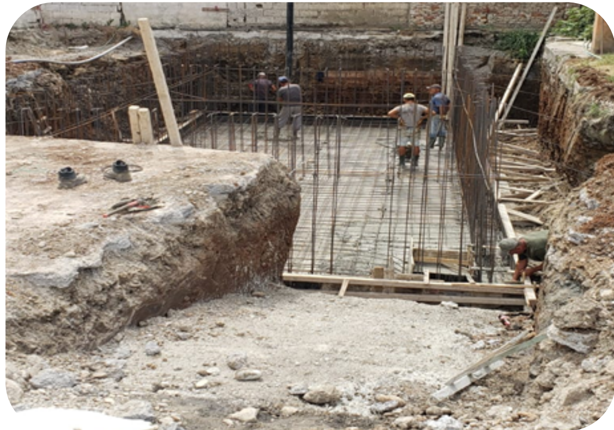
2 underground tanks with a total capacity of 70 m 3
